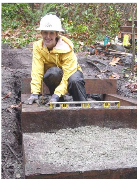
Constructing box steps, with a level and a smile, in Seattle's Ravenna Park.
